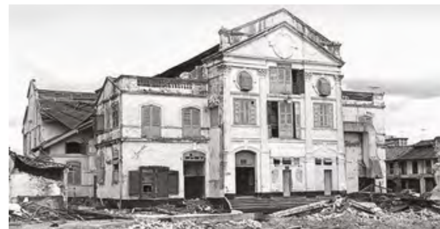
Theatre Royal in the midst of demolition in 1977. Image reproduced from Remember Singapore website.
